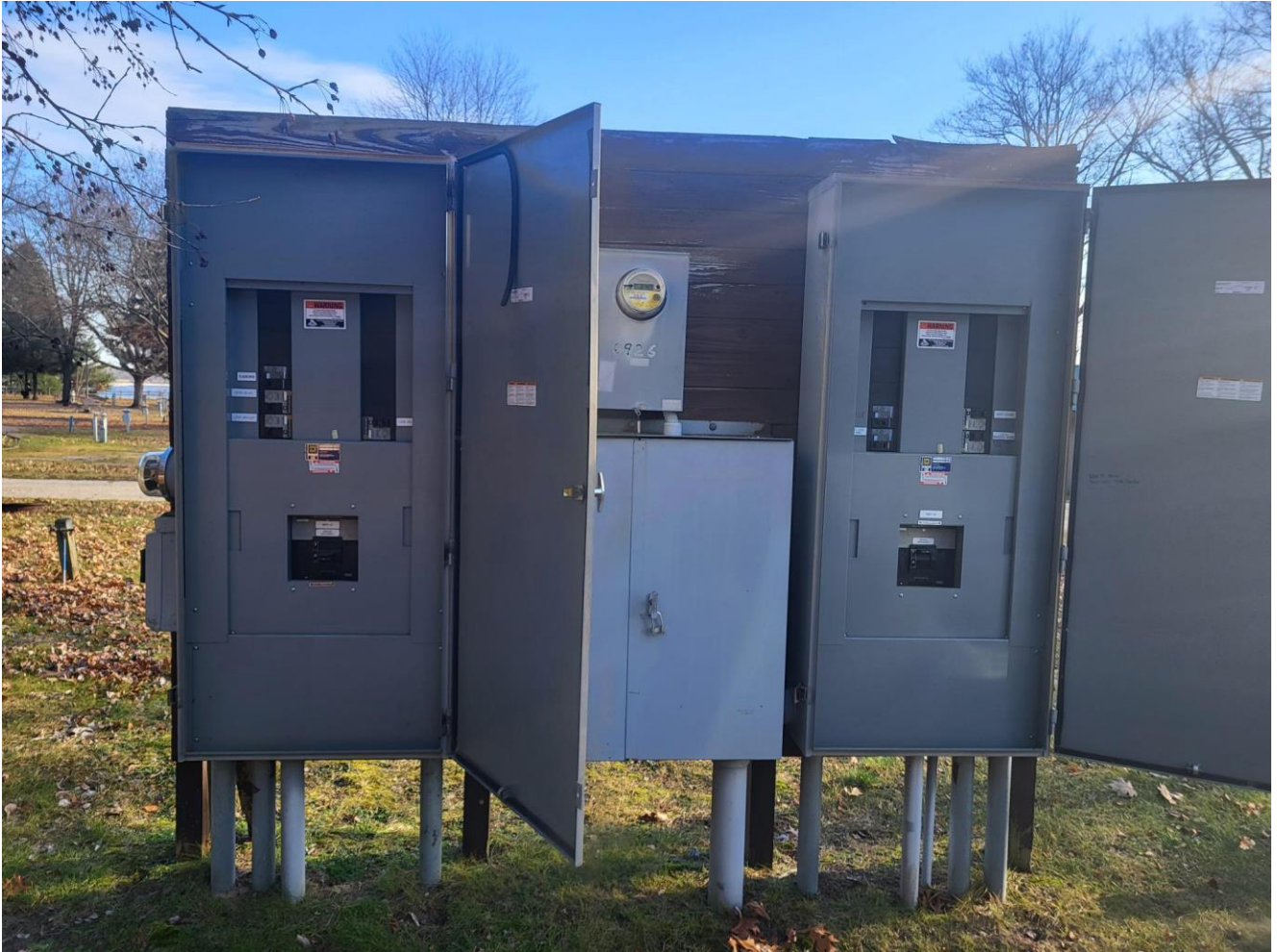
Main pannels near site 1 Two 600amp pannels
